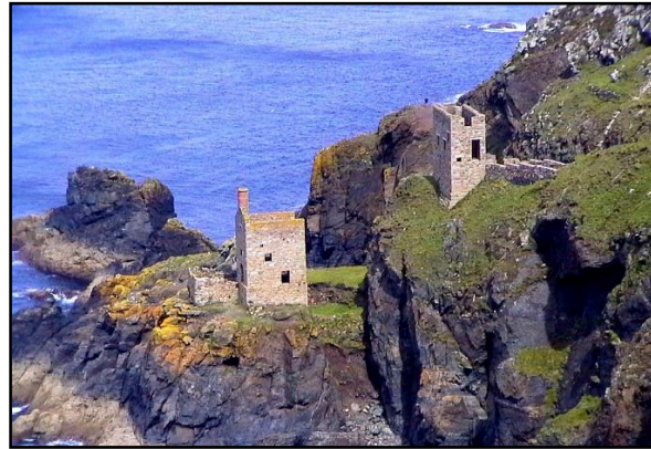
The 1984 stabilisation project for the Crowns Engine Houses at Botallack led by CBMS was, at the time, the largest scheme of its type ever carried out by a private group.
